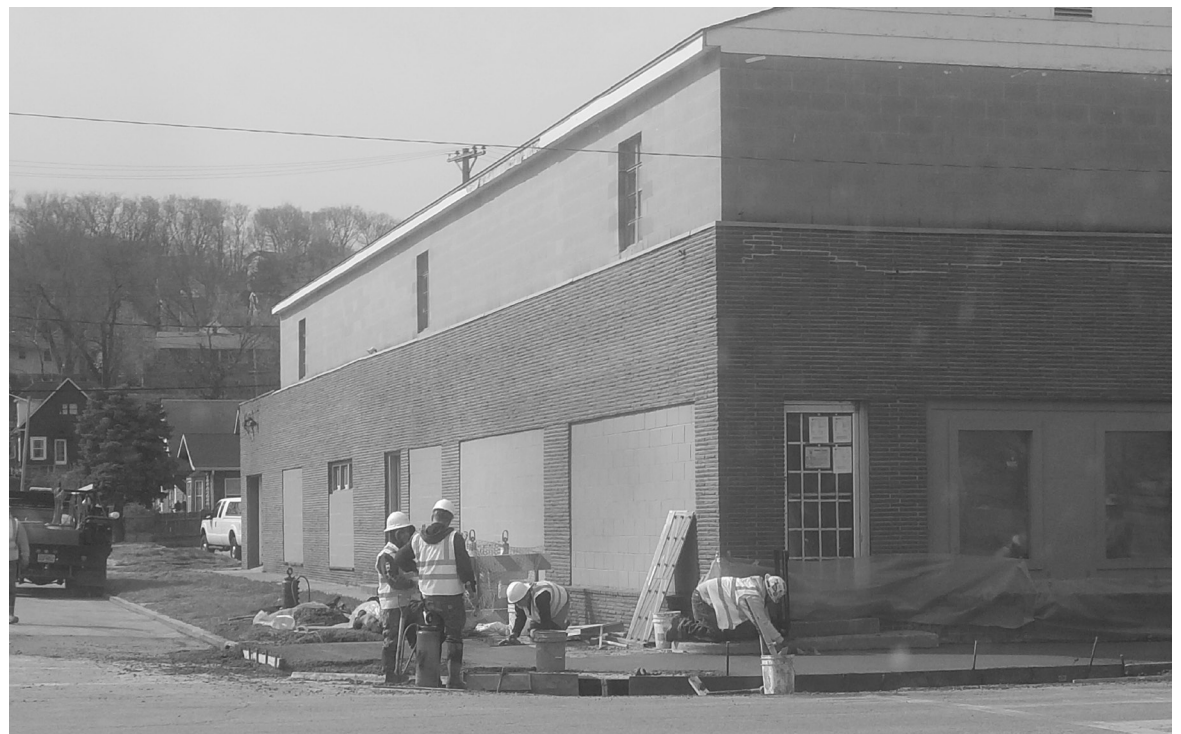
This is a team of workers getting some much-needed work done since the weather is permitting.
