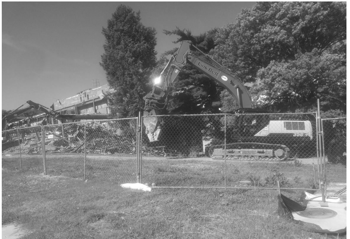
This was the original Turner High school then it became Turner Middle school. It is being razed and rebuilt.
