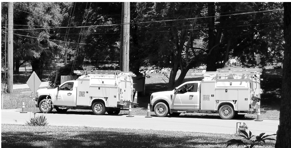
Two trucks checking the big electrical boxes. At least some people are working.
