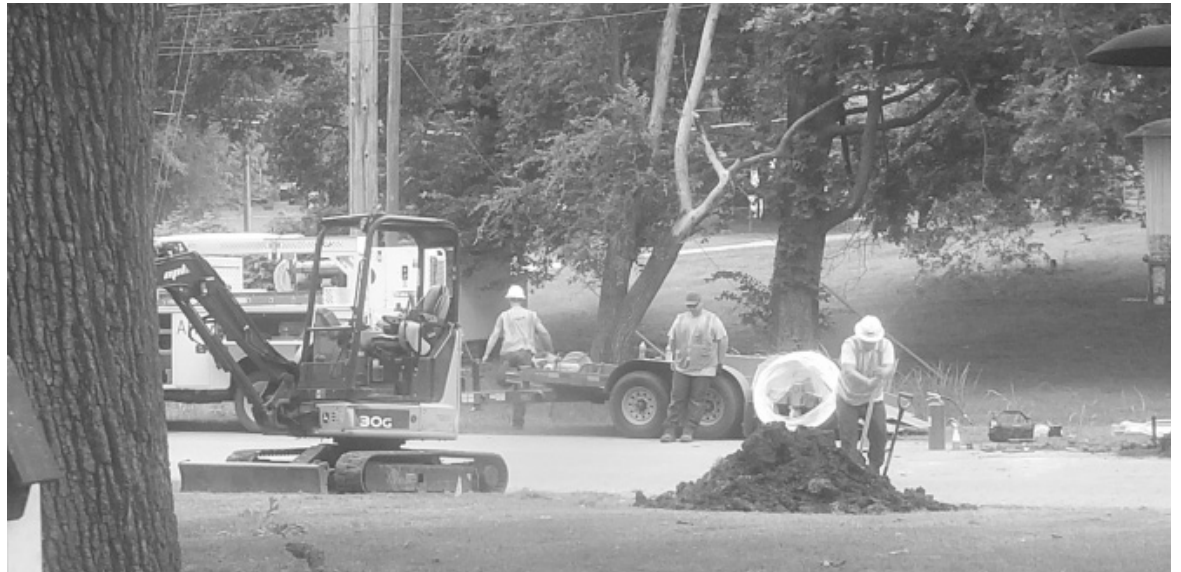
These men are working diligently on the street. They are going to put in a new meter further away from the street.
