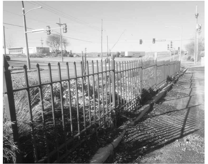
A wrought iron fence is being erected around the parking area of the community garden in Turner. Thanks so much to Josh Markley for getting it for us. We do have some wonderful people in Turner.
